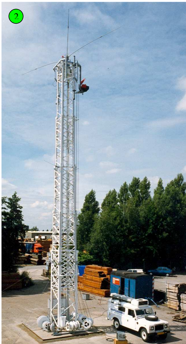
20 m GTM, fixed installation
